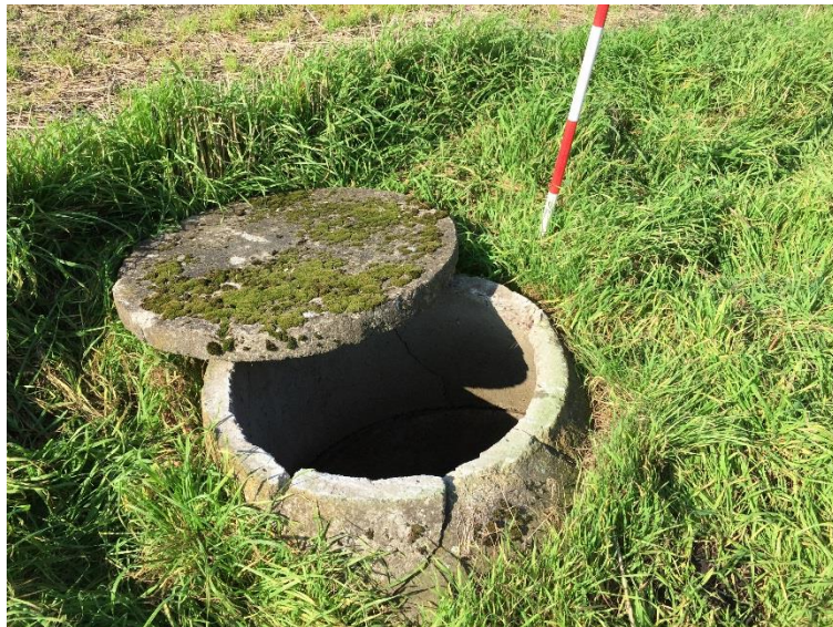
Figur 6: Brønd i afvandingsystem 7.
